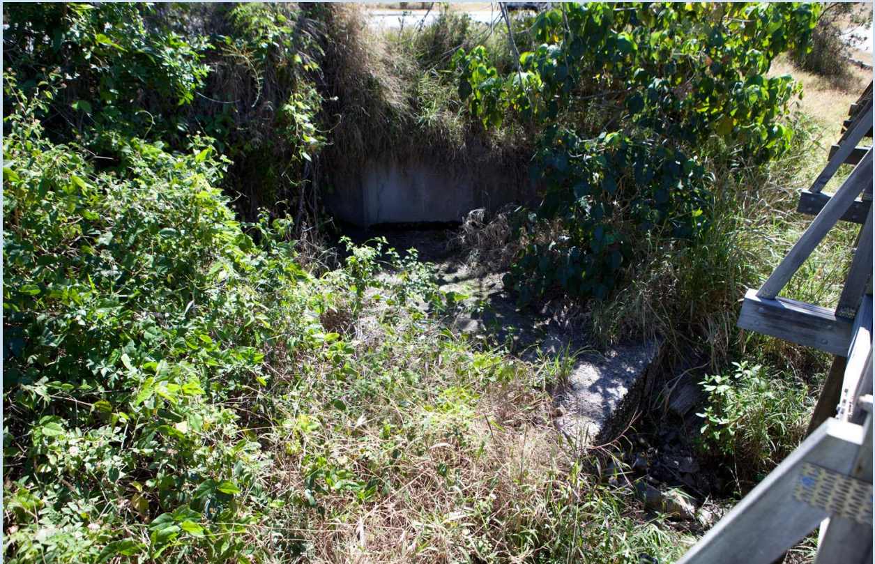
Marcus Creek at David Low Way (MCS 2) – Single Culvert crossing with significant 'drop-off' causing fish passage restriction and stream bed erosion.
