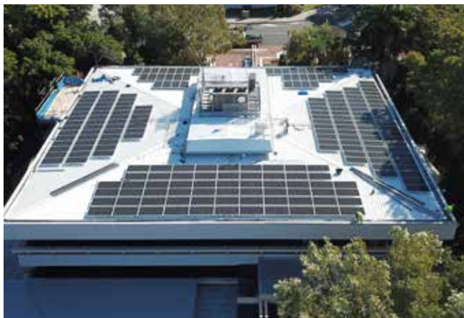
Solar installation at Tewantin administration building
