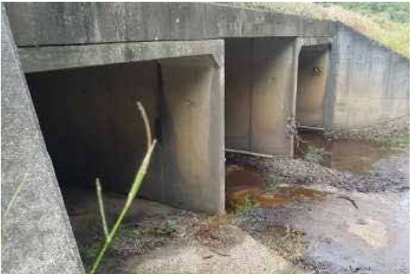
Culvert barrier to fish passage
