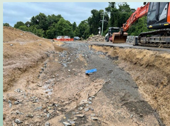
Damage to construction
