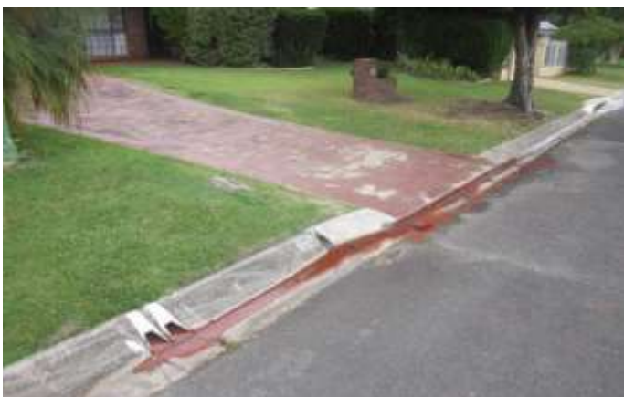
Wastewater residues left in a roadside gutter
