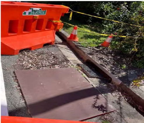
Damaged stormwater area
