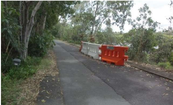
Damage viewed from the road
