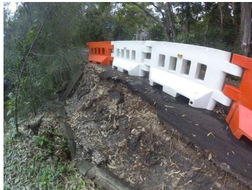
Damage viewed from the river
