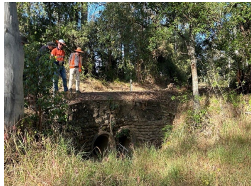
Damaged culvert near Schreibers Road on Coles Creek Road.
