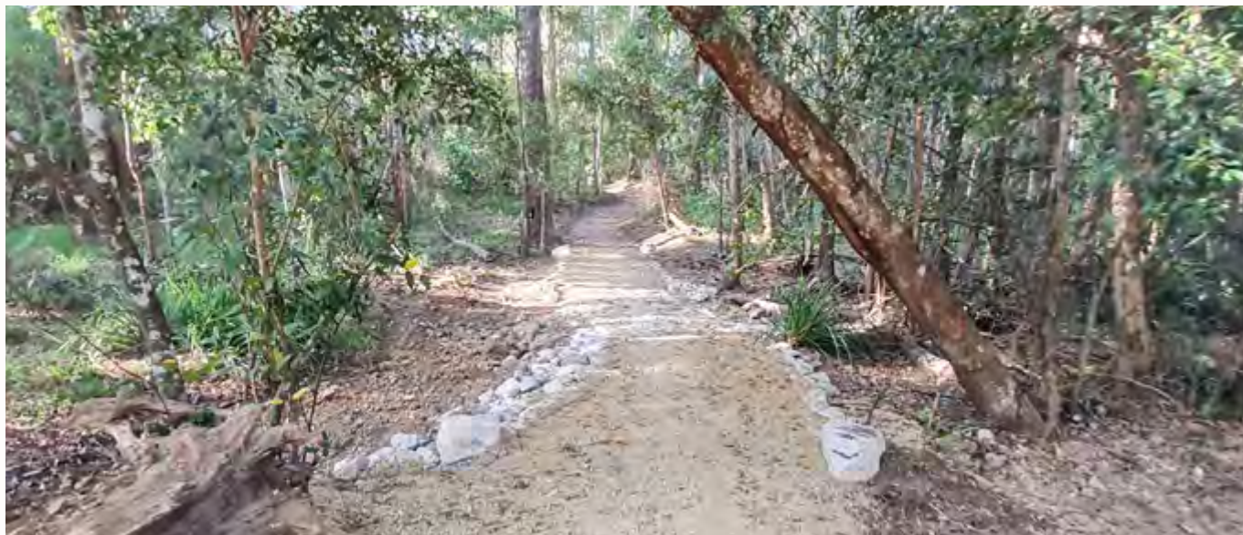
Recent upgrades to Trail 5 of the Noosa Biosphere Trails (image source Aiden Flannery).
