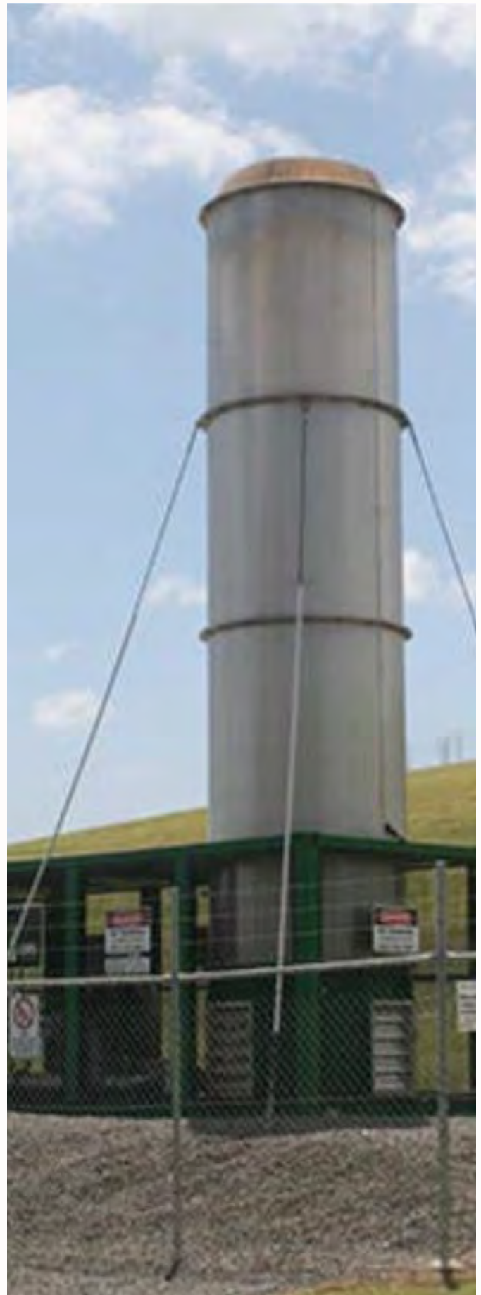
Methane gas extraction well at Eumundi-Noosa Road Resource Recovery Centre
