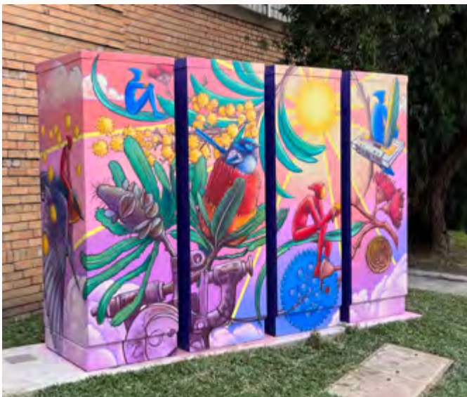
Example of a community battery - Fitzroy North Community Battery (image source YEF 2023)
