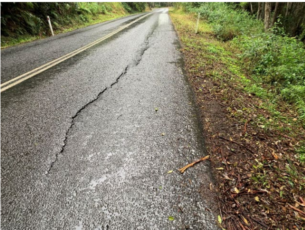
Pavement damage from landslides on Cooroy-Belli Creek Road
