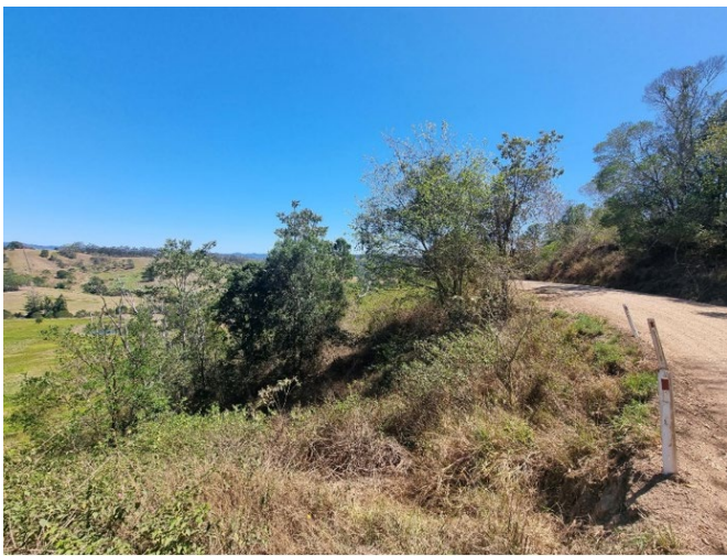
Site of damage on Happy Jack Creek Road looking north.
