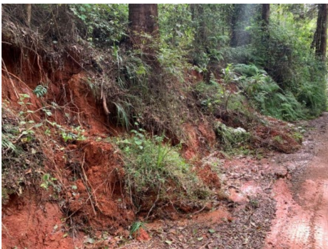
Damage to the slope on Old Ceylon Road
