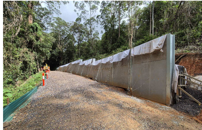
Main retaining wall structure reaching up to 4m above the existing road.
