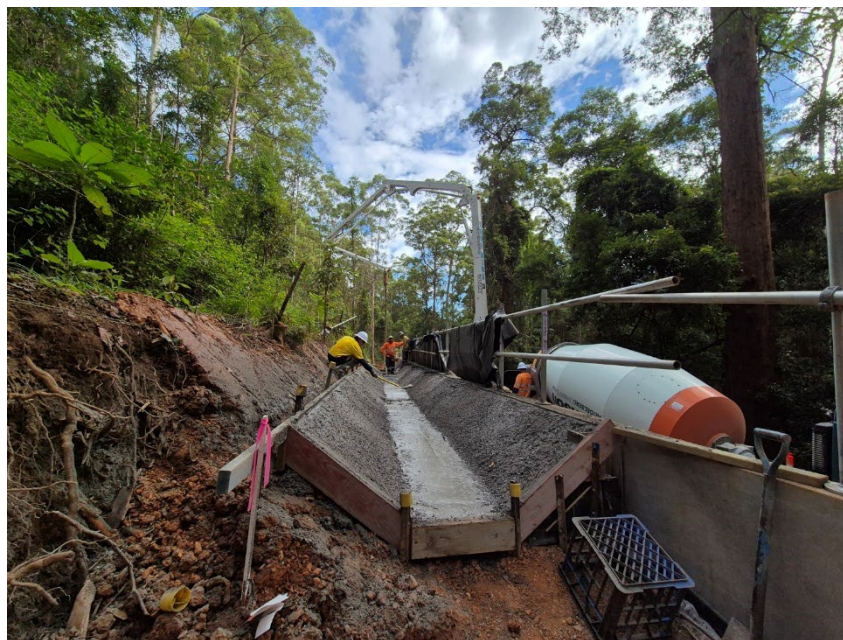
Putting in the shotcrete drain at the top of the retaining wall.
